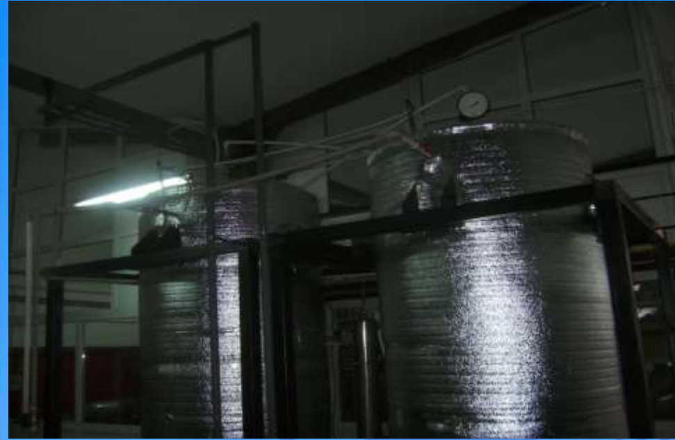
Front view of the pilot installation
