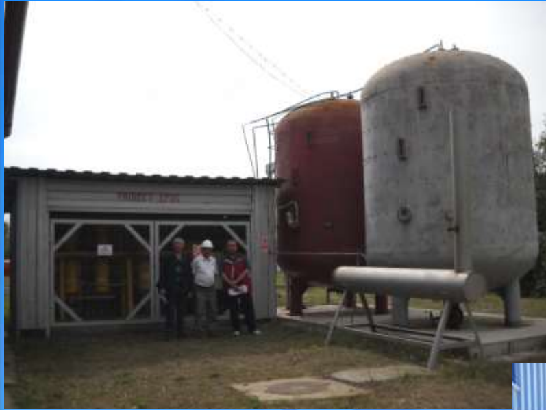
Overview of the pilot installation
