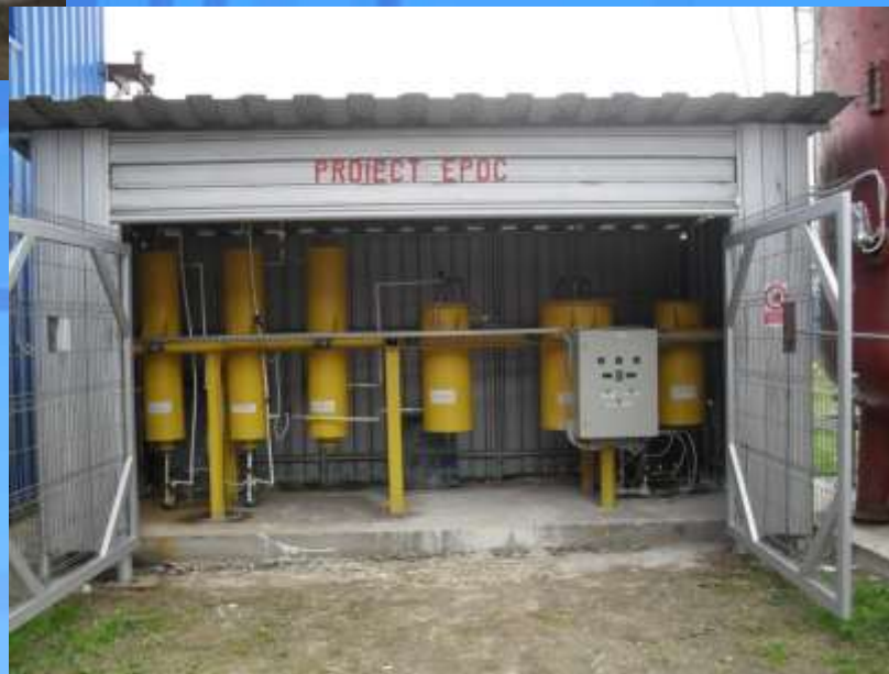
Front view of the pilot installation
